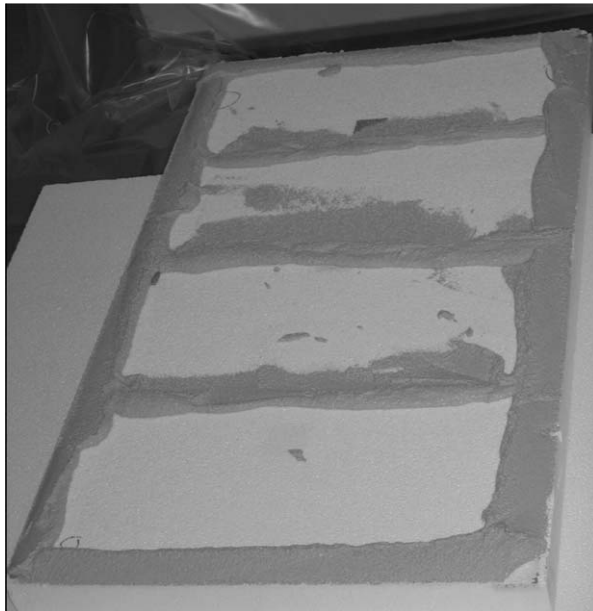
Fig. 6. Plaster stripes on the insulation board to glue it onto the concrete wall.
